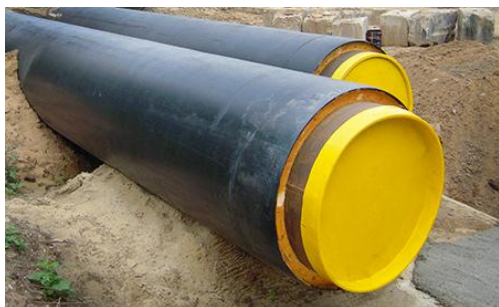
Figure 4. PPU pipes for heating and water supply (heating).
