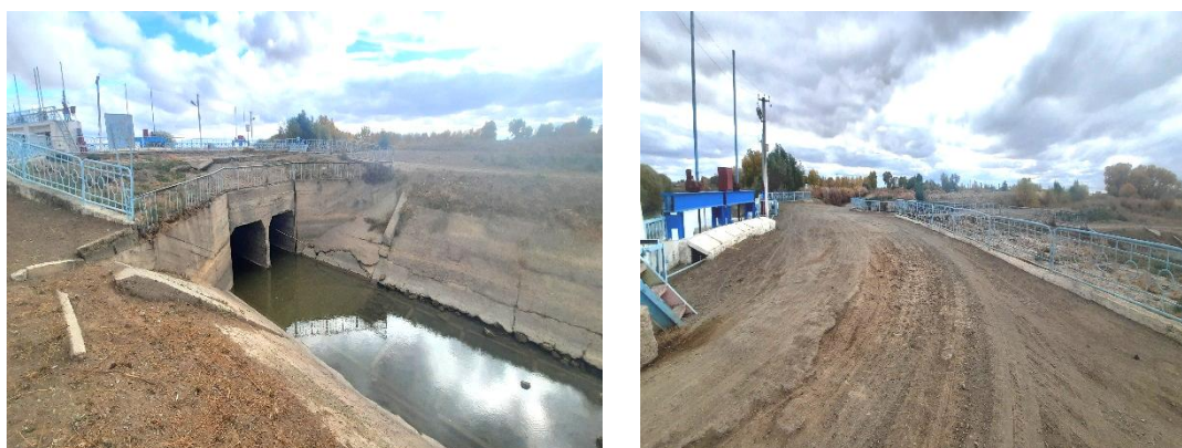
2-rasm. Inshoot texnik holatida yuzaga kelgan deformatsiyalar Figure 2. Deformations arising in the technical condition of the structure
